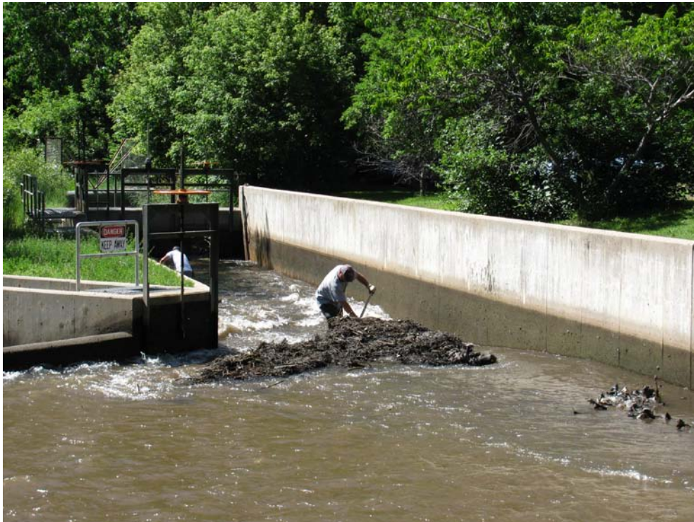
Figure 1 Clean-out operation and Debris
